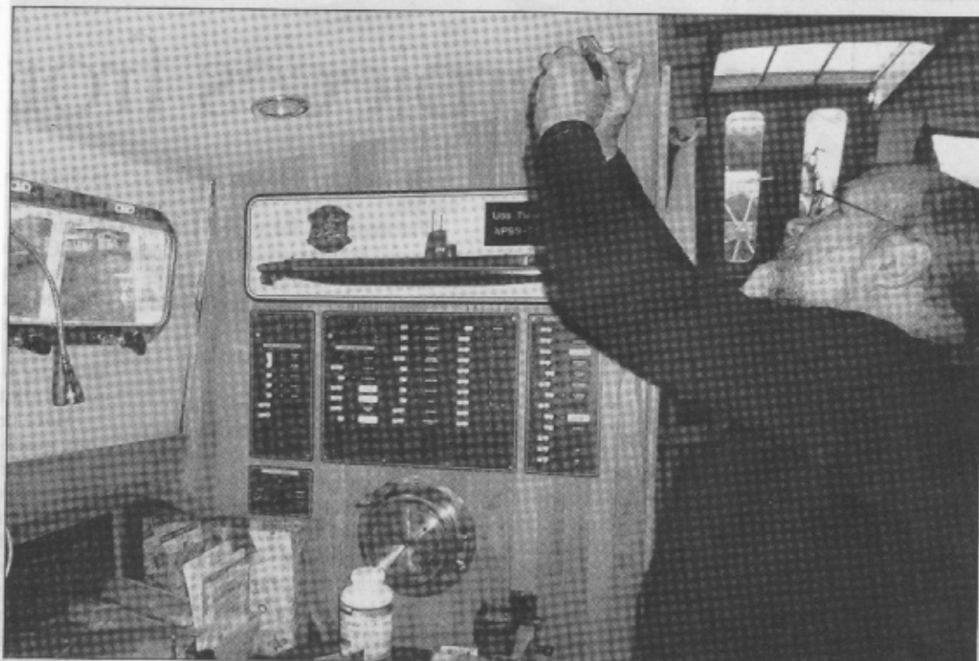
Greg Kerkof installs light fixtures above the roll-top desk in the main salon. Kerkof served on USS Tunny when he was in the Navy.
